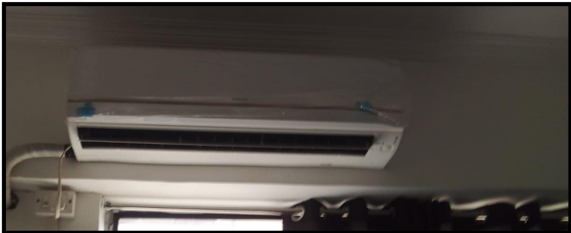
Split AC Indoor Unit
